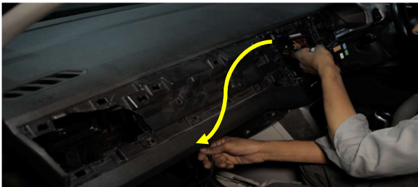
STEP 25 :- ROUTE SAVV DEDICATED POWER CABLE (PART 9 ) FROM THE BACK OF THE MULTIMEDIA/INFOTAINMENT TO GLOVE BOX AREA AS SHOWN
