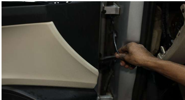
STEP 83 :- ROUTE CABLES AS MARKED (KINDLY REFER TO THE VIDEO IF ANY CONFUSION)
